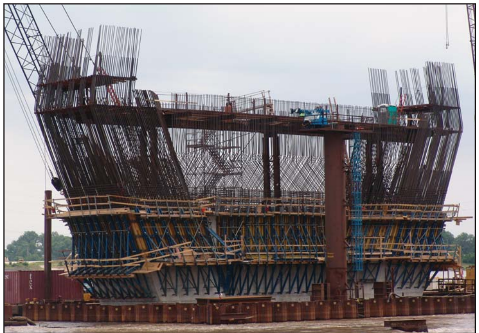
Reinforcing steel on the river tower on the Missouri side takes shape.
