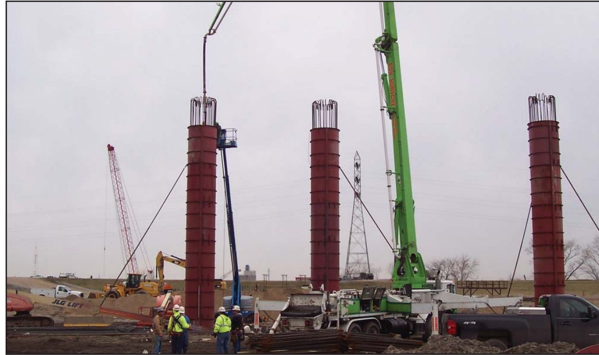
Construction on the Illinois Approach continues. Here, crews place concrete in the columns that make up a portion of the bridge foundation.
