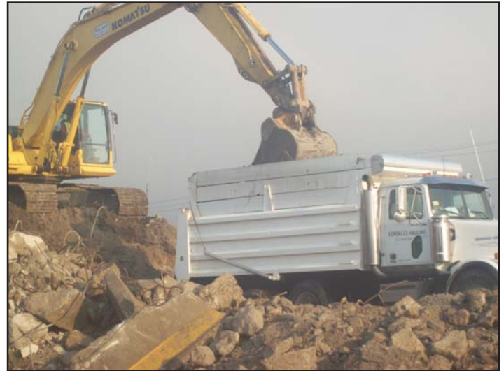
Kendall Davidson, a Disadvantaged Business Enterprise owner-operator, hauls material away from the Missouri Approach project. Davidson is a graduate of MoDOT's Supportive Services Fast Track program.
