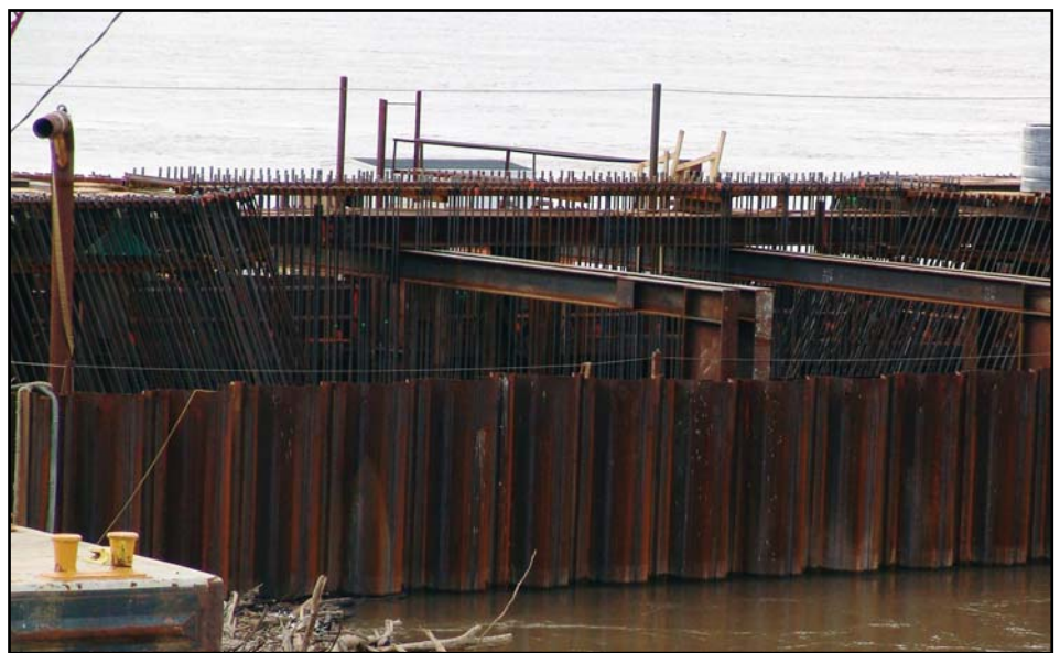
Steel for the Illinois tower rises out of the Mississippi River. Crews will be working on the 400-foot towers for the next 18 months.
