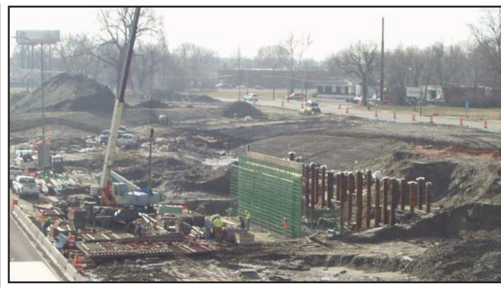
Workers build retaining wall for the 15th Street bridge over Interstate 64 in Illinois.
