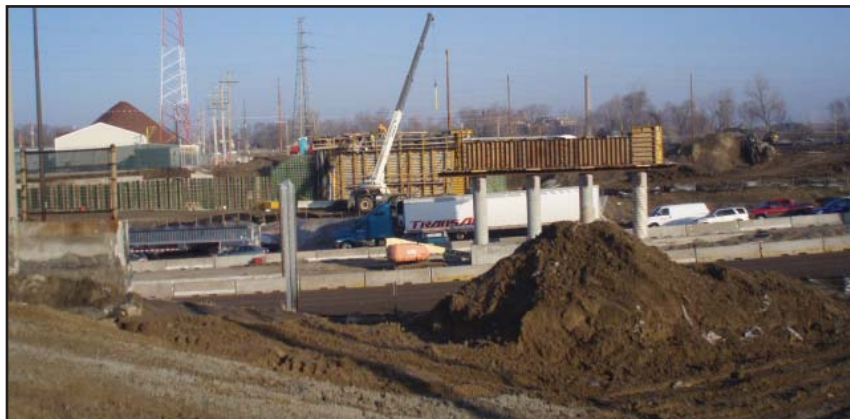
The construction team pours a foundation cap for the Exchange Avenue bridge in Illinois.
