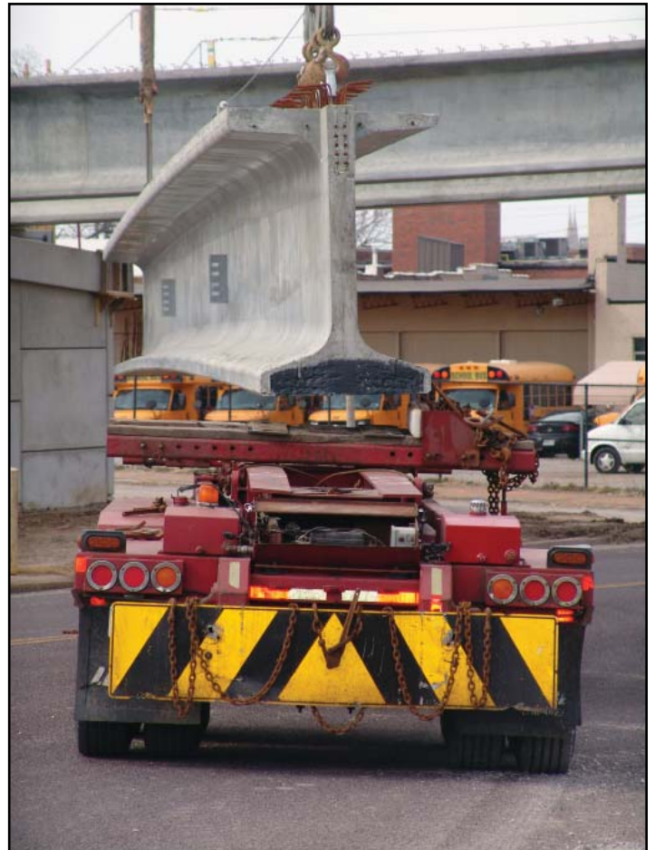
The tractor trailer maneuvers the girder into place so a pair of cranes can lift it into position.
