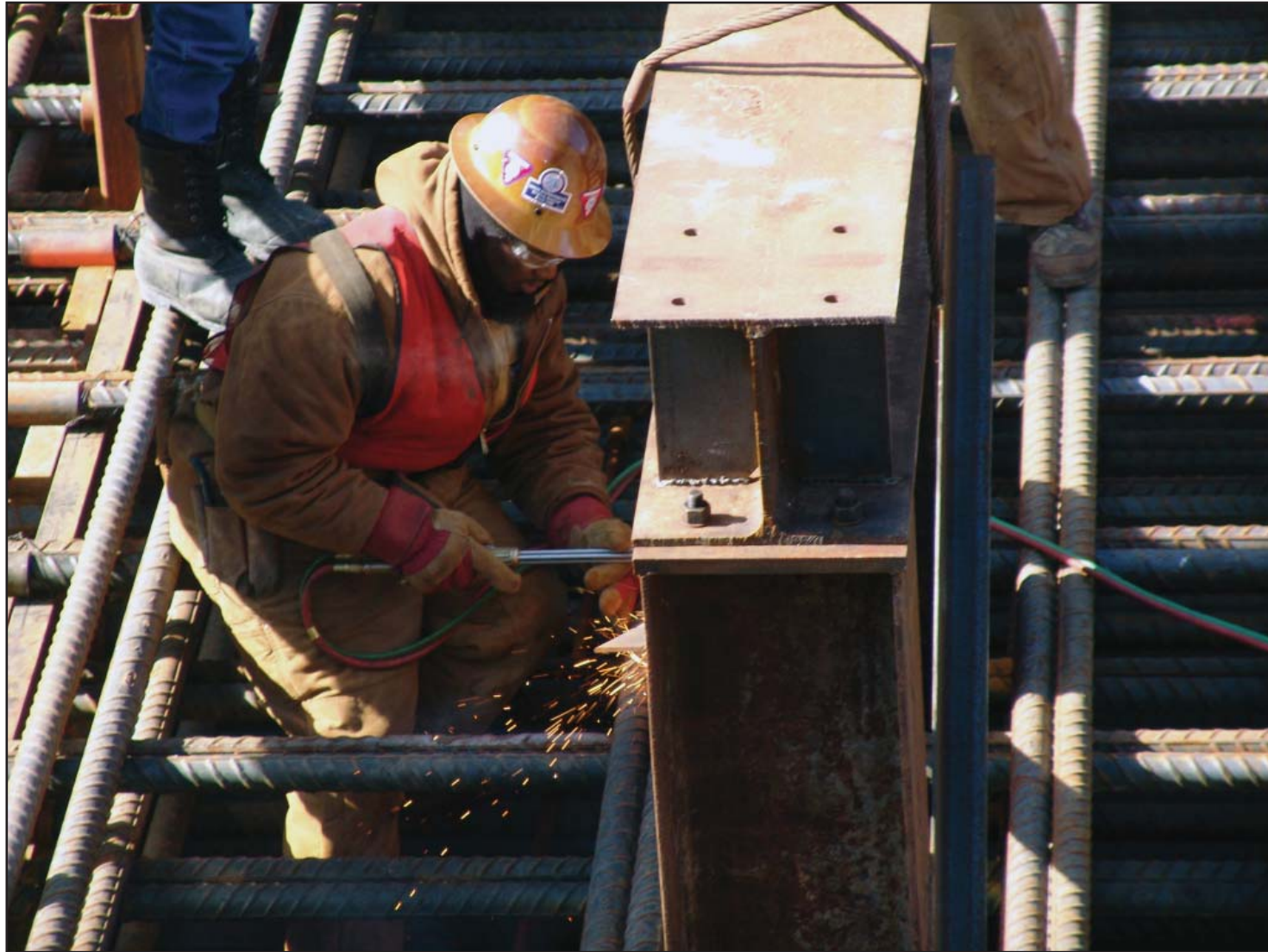
An ironworker installs a portion of the steel framework for the Illinois river tower foundation
