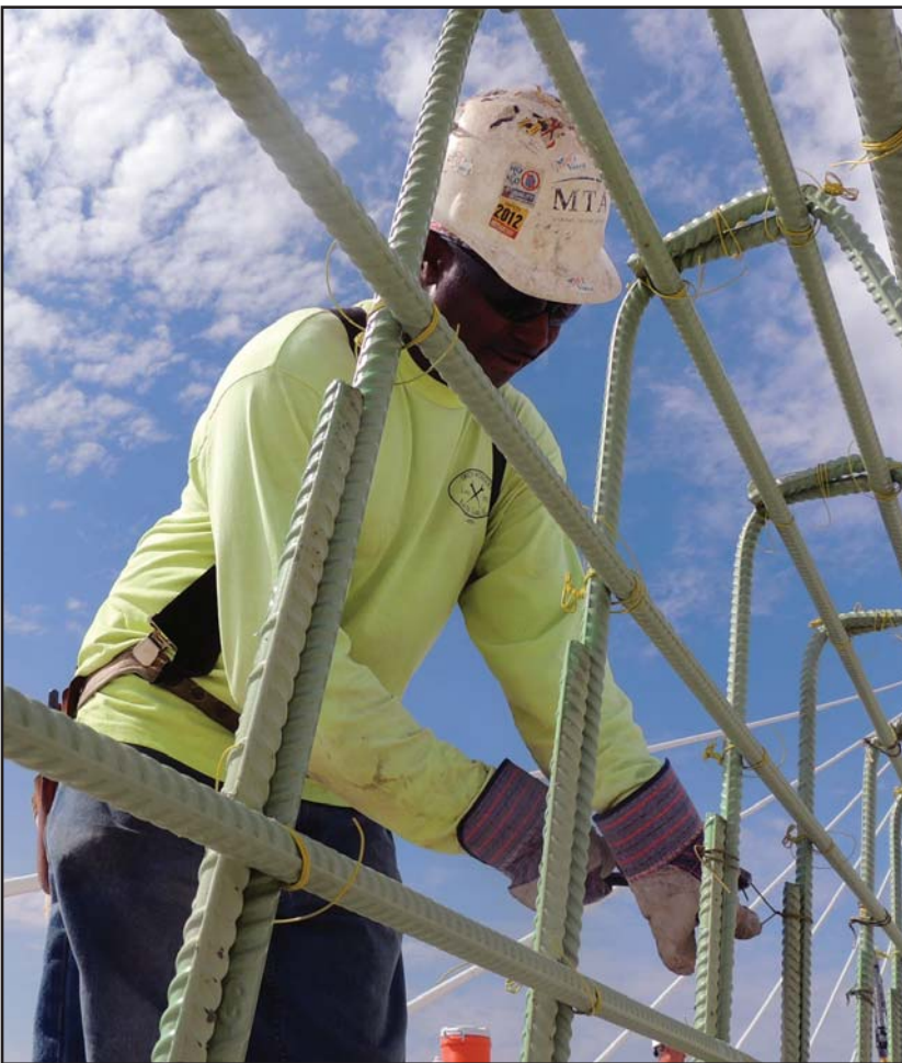
An ironworker ties together reinforcing steel for the barrier that separates eastbound and westbound traffic.
