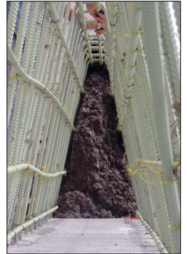
Concrete is forced inside and around the steel to form the middle barrier.
