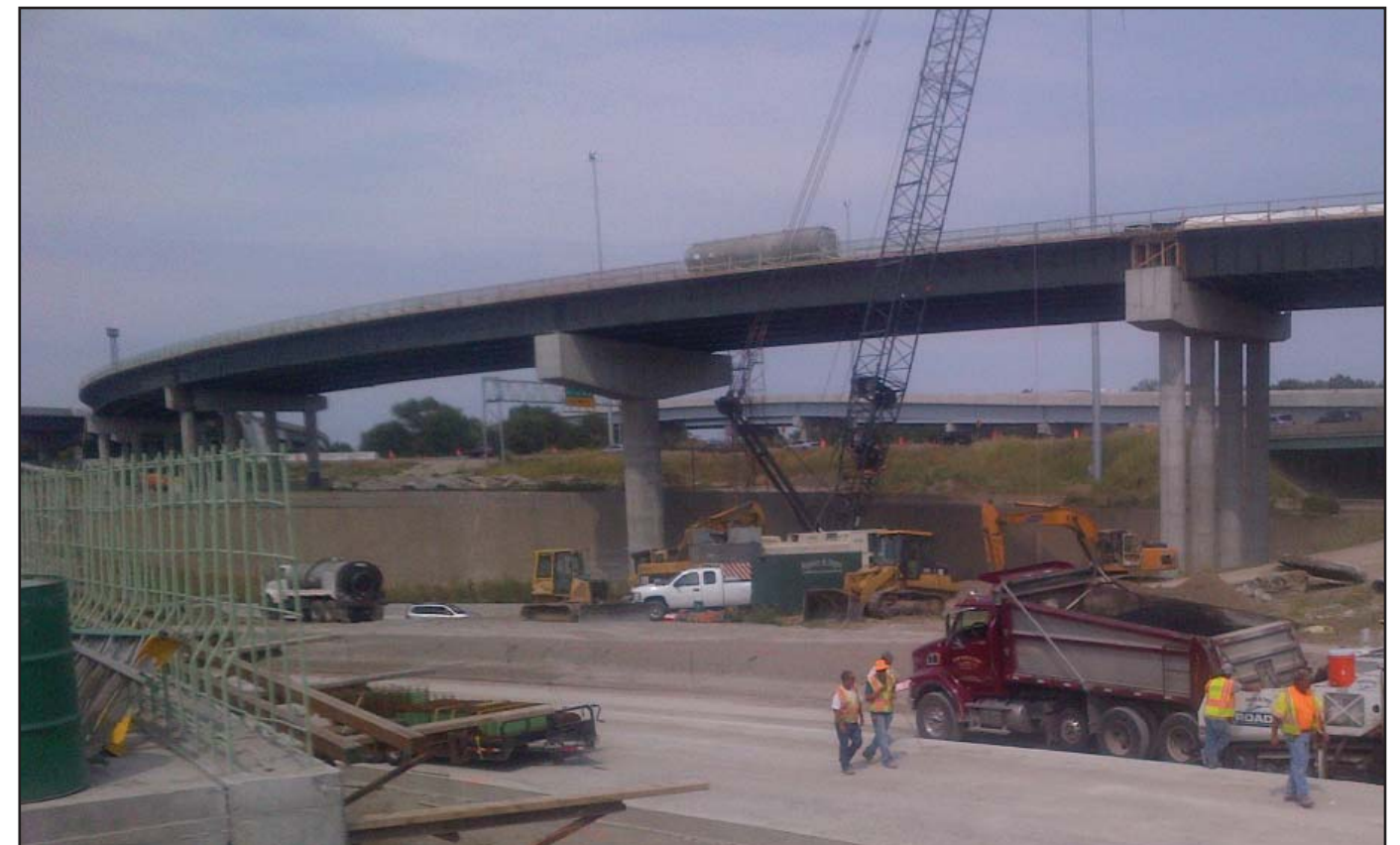
Crews work in Illinois finish the construction connecting existing interstates to the bridge.
