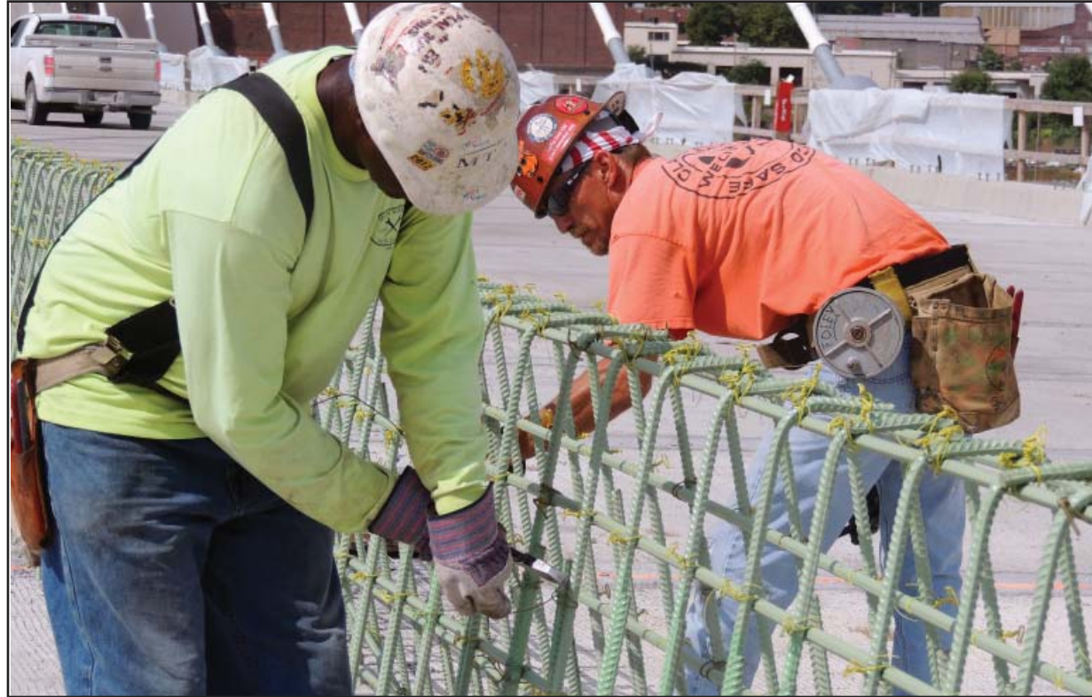
Ironworkers tie the steel for the concrete barrier across the middle of the bridge.
