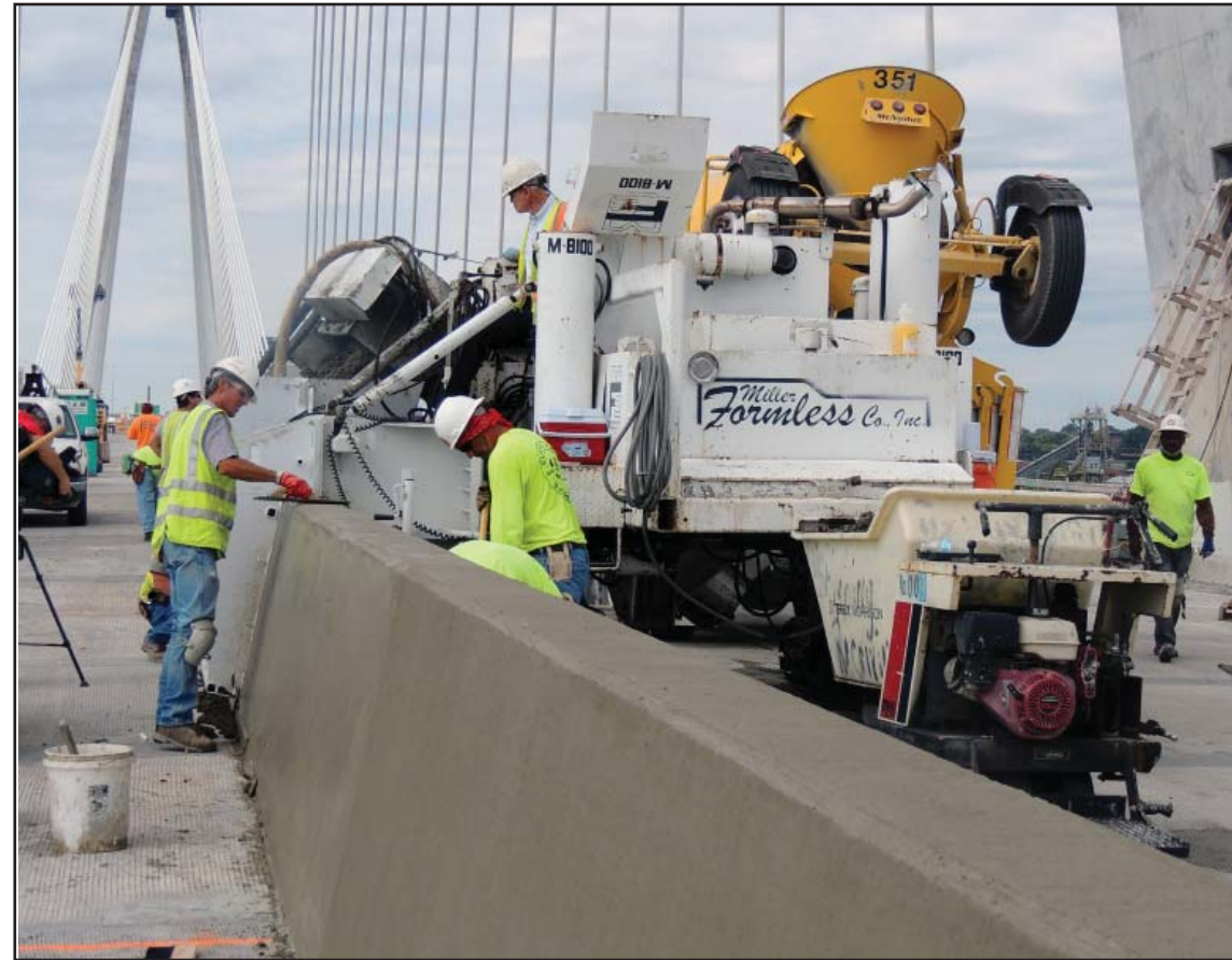
Concrete crews build the middle barrier using a process called slip forming.
