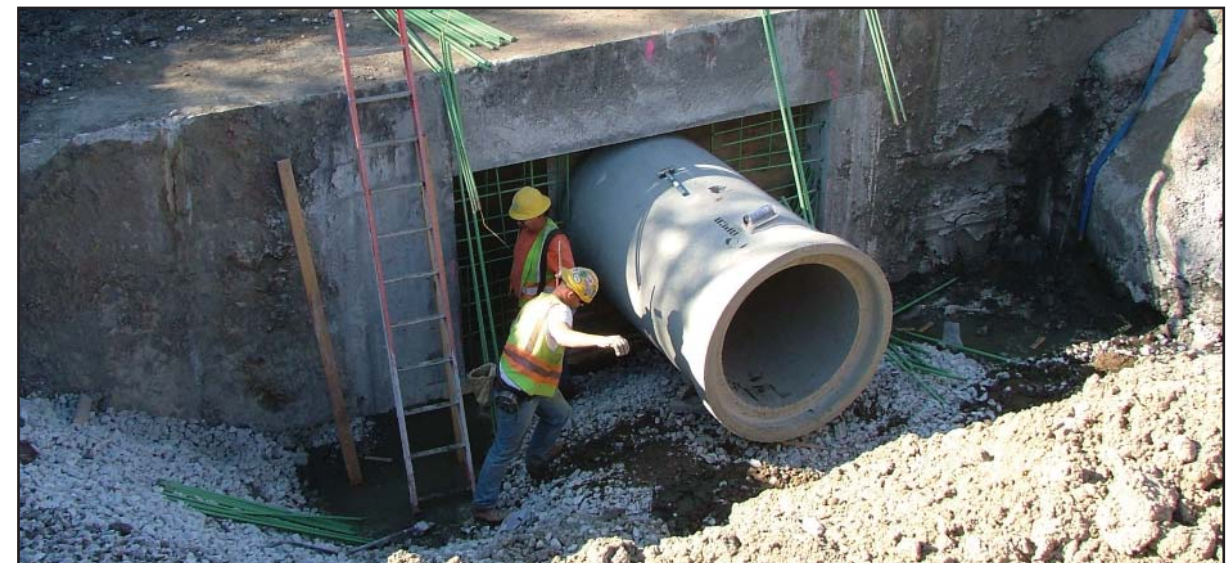
Utility crews relocate water lines as part of the efforts to relocate Interstate 70.
