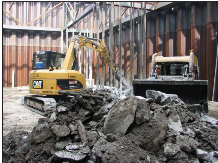
Operators break up and remove the concrete from the floor of the Mississippi River inside the Illinois cofferdam.
