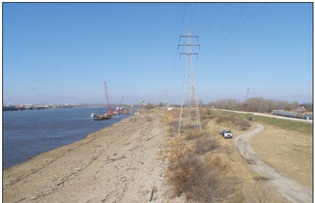
A shot of construction on the Illinois side of the Mississippi River from the new construction camera.
