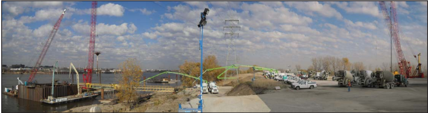
Concrete trucks line up to pour nearly 3,000 cubic yards of concrete for the seal course, part of the foundation for the river bridge project. The seal course gives crews a flat, solid building surface on the river bottom.
