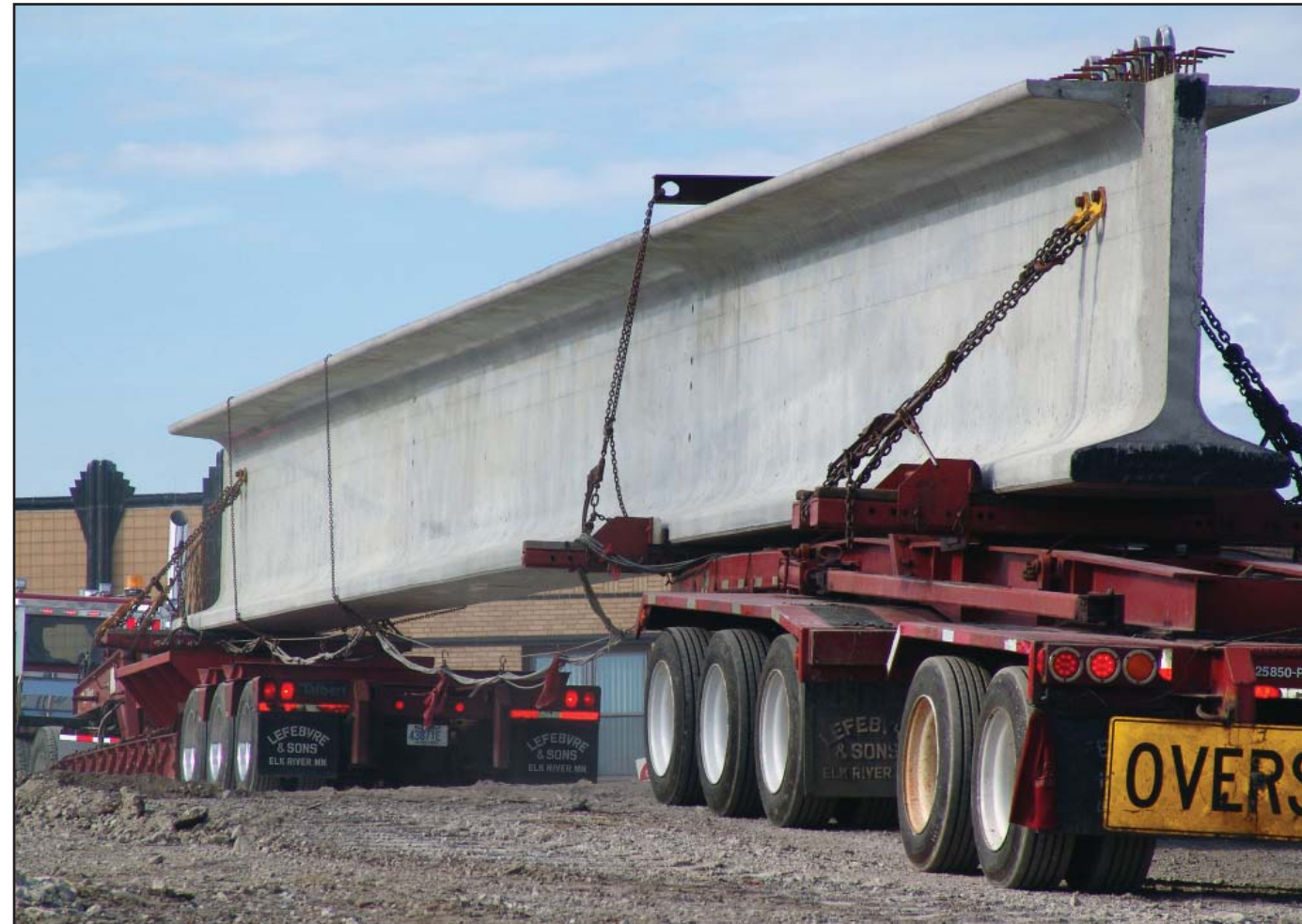
A driver backs one of the massive girders into position to get lifted into place.
