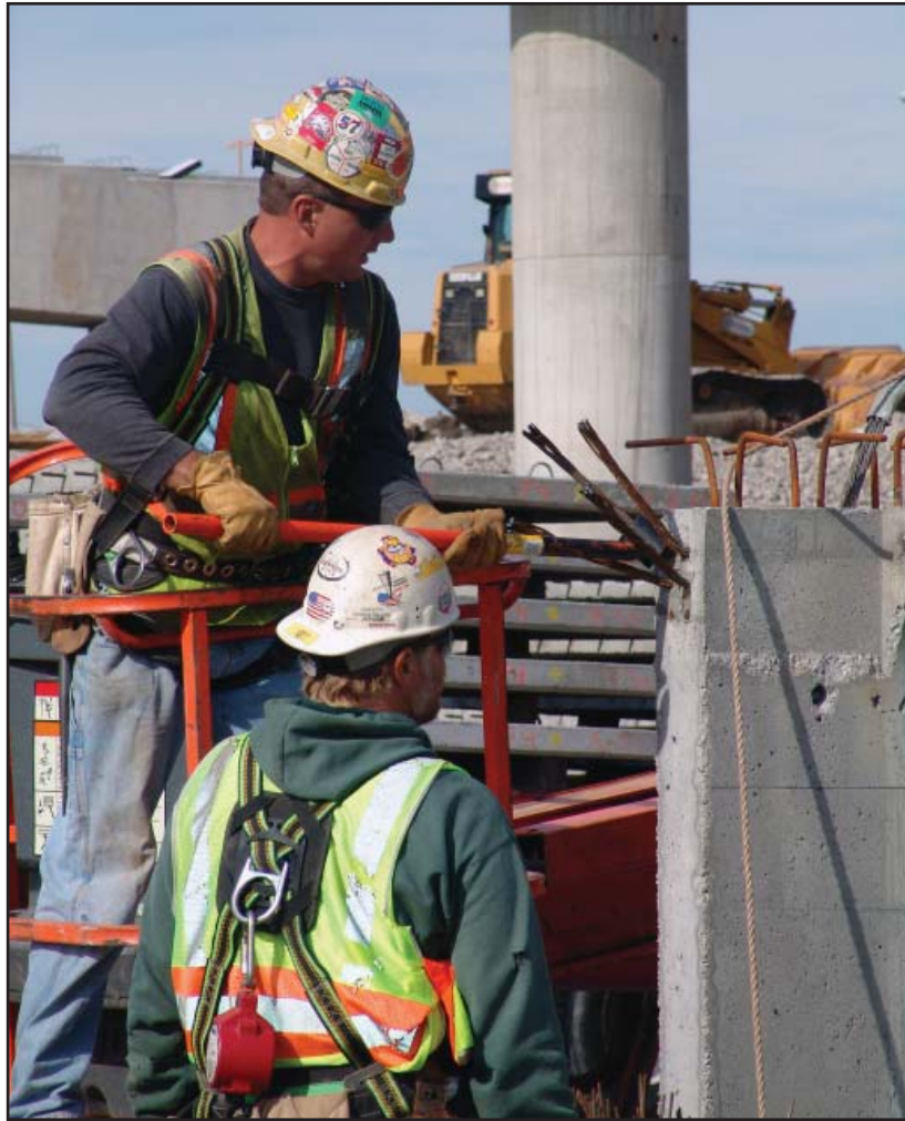
Workers straighten reinforcing steel on a girder before placing it on the Missouri approach.
