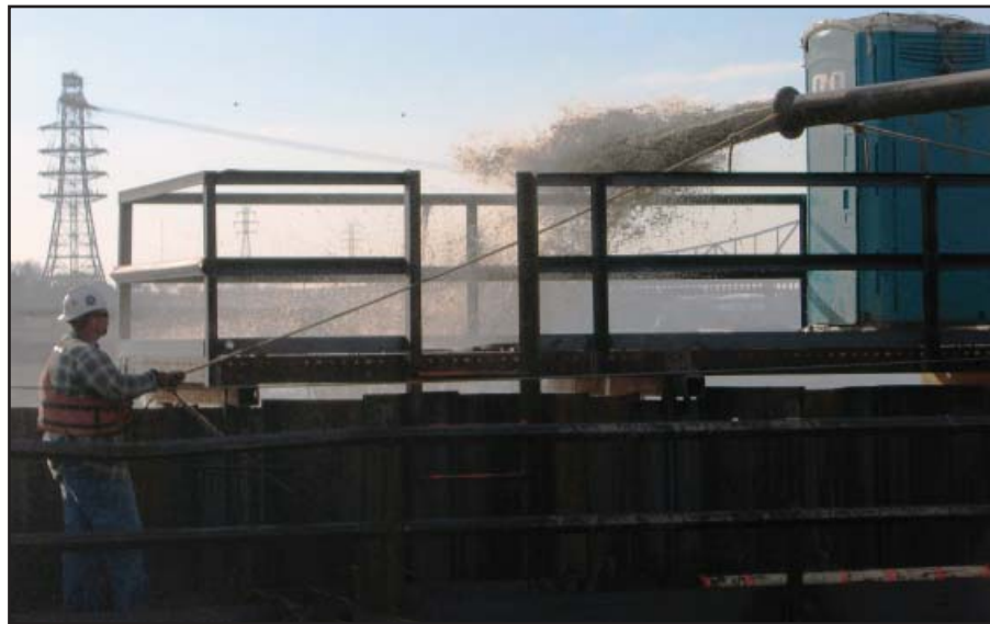
Crews use a pump to remove water from the cofferdam while pouring 3,000 yards of concrete.
