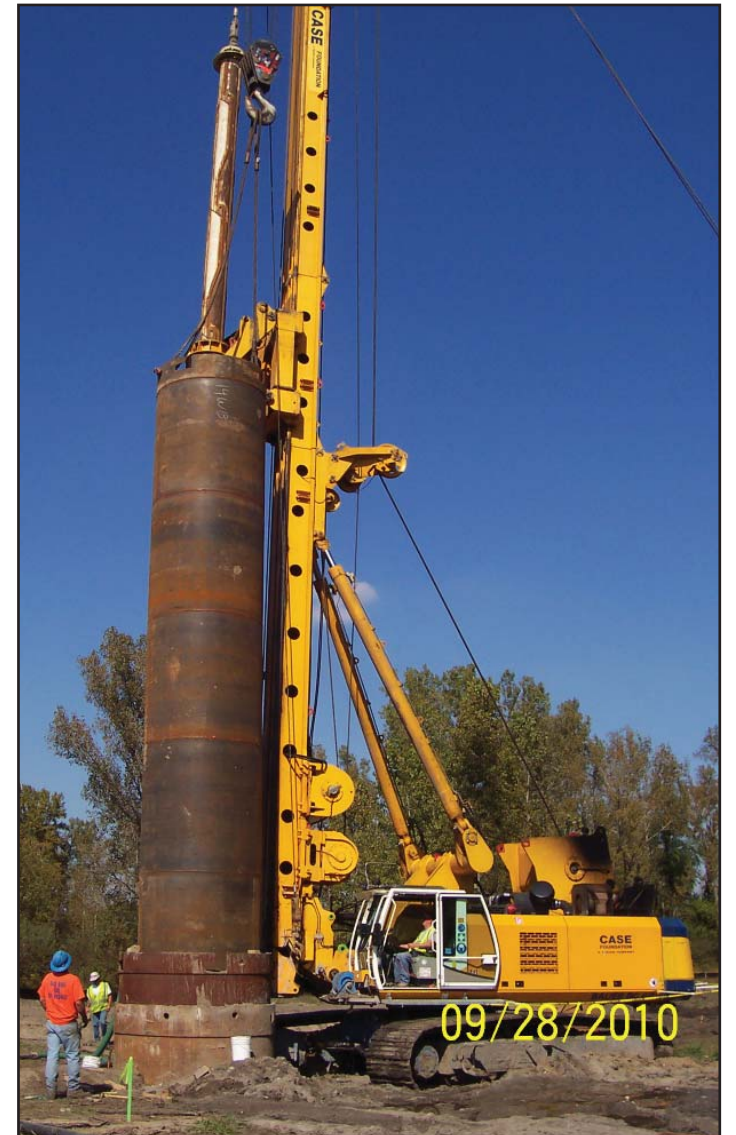
Equipment operators drive a casing into the ground for the Illinois approach.
