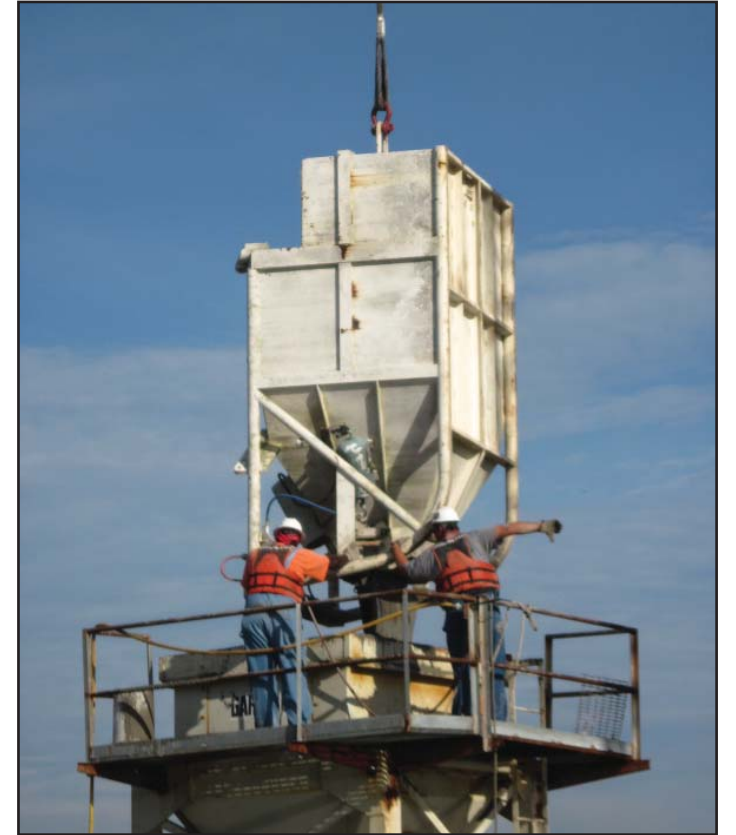
The contractor pours concrete into the shafts for the main span of the bridge.
