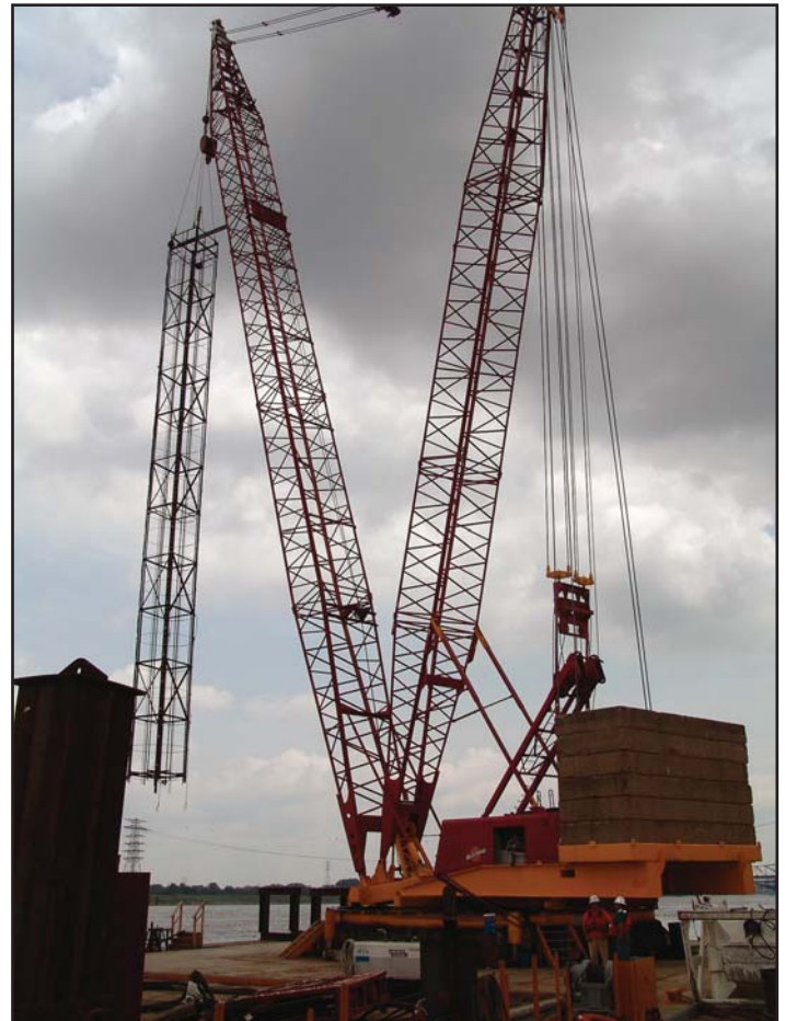
A crane moves the load test framework before welders attach the hydraulic cells.
