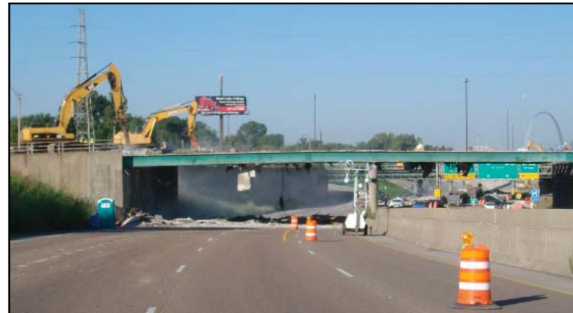
LEFT: Workers slowly lower the rebar needed to support the main span foundations into shafts drilled into the river bedrock. As the rebar is lowered, welders attach rebar circles to help the rebar maintain its shape. ABOVE: Multiple trackhoes remove a portion of the Exchange Avenue bridge over Interstate 55/70. The bridge needed to be removed to prepare for a new I-70 connection to the main span of the bridge.
