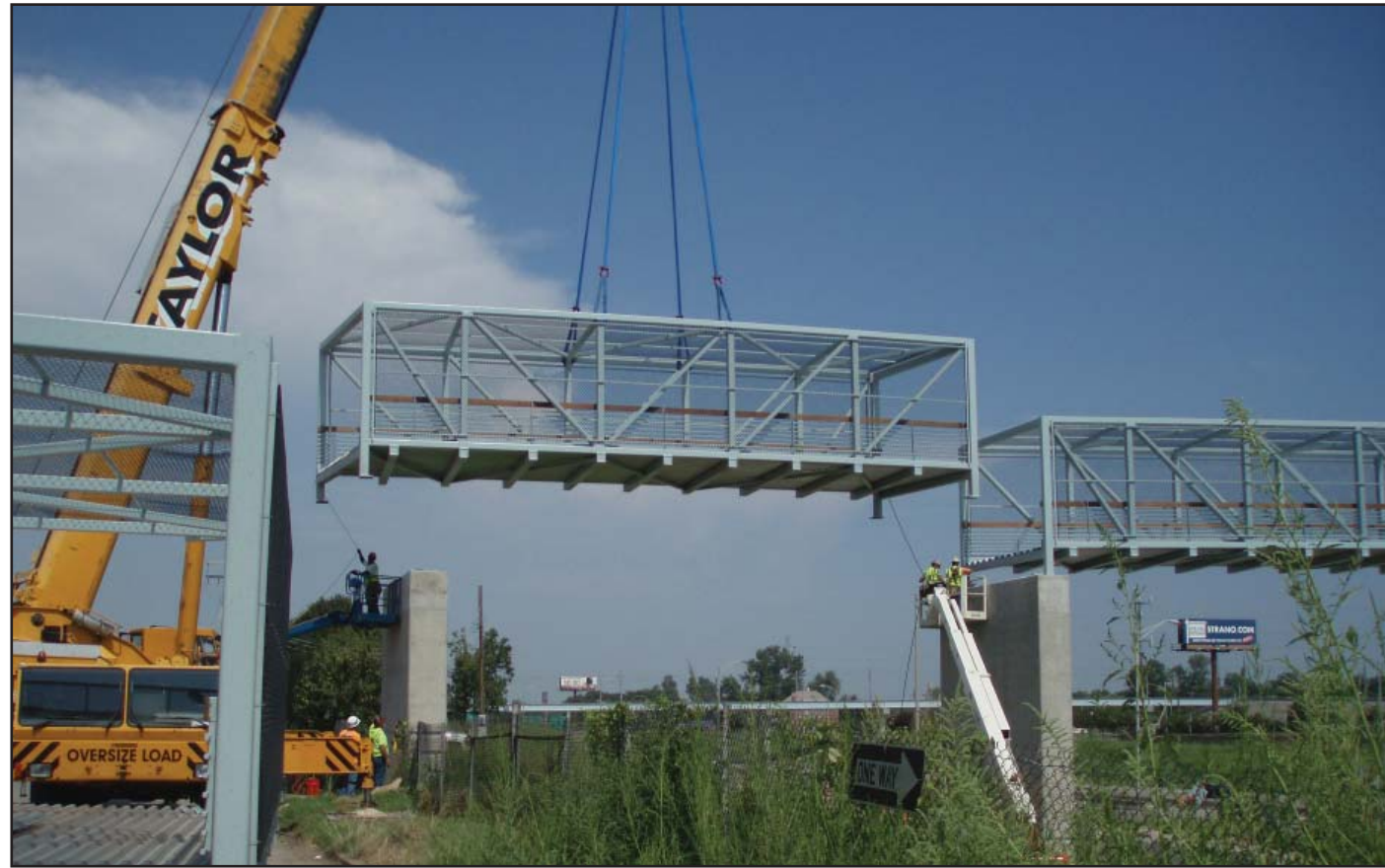
Illinois crews move a portion of the pedestrian bridge over I-64 into place.
