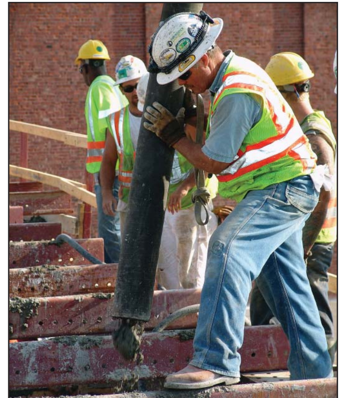
Fred Weber Inc. workers pour concrete for the largest cap for the Missouri Approach. The roadway will rest on this cap.
